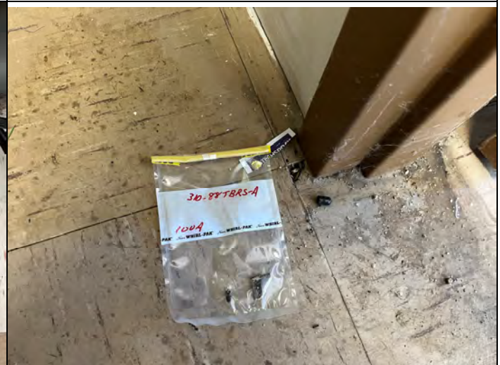
Photo 10 – Sample 310-88TBRS-A, ACM 12" tan w/ brown streaks floor tile in building 88, room 100A. Both the tile and mastic contain.
