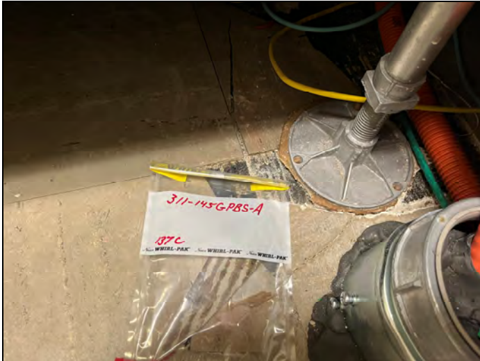
Photo 7 – Sample 310-145GPBS-A, asbestos containing 12" gray with pink and black streaks floor tile and black mastic in building 145, room 137C. Both tile and mastic contain.
